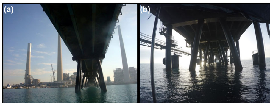
FIGURE 2 Hadera infrastructure site: Orot Rabin Power Station coal conveyor and jetty infrastructure above water and under the conveyor. (a) Coal conveyor piles. (b) Coal jetty piles
